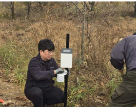
Installation of Data Logger and Temperature/Humidity Sensor
